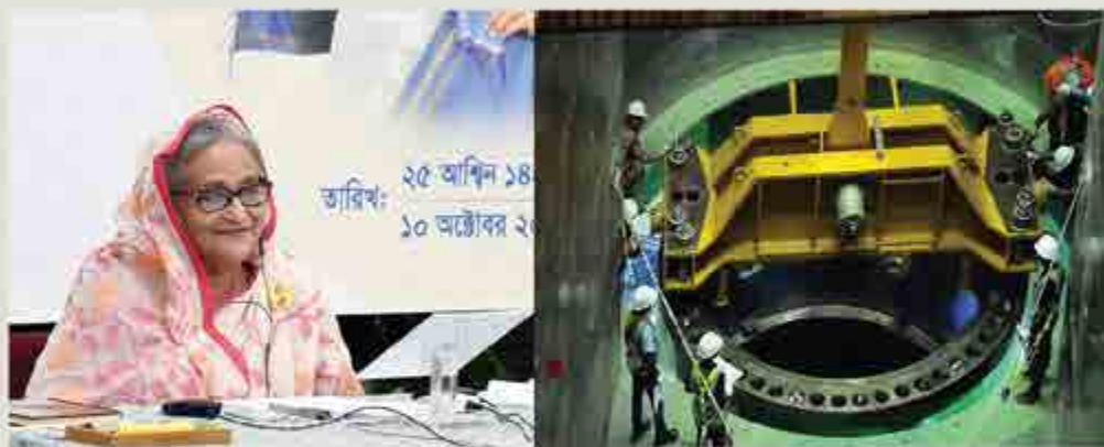
Prime Minister Sheikh Hasina, joining virtually from her official Ganobhaban residence in Dhaka, inaugurating the reactor pressure vessel-installation work of the first reactor building of the Rooppur Nuclear Power Plant Project on October 10
