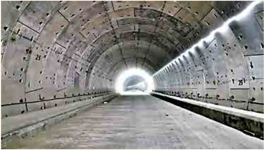
Bangabandhu Sheikh Mujibur Rahman Tunnel, Chattogram- the only under water road tunnel of Bangladesh
